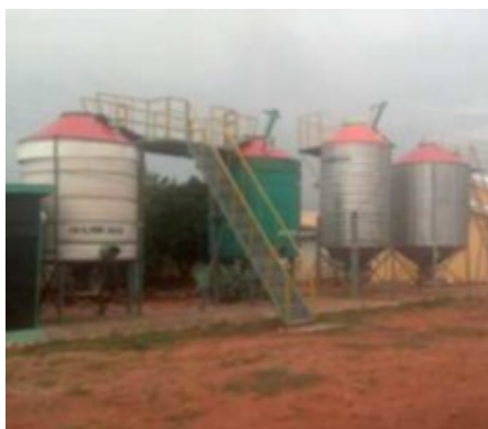
Solar Aeration Storage Silos at PENS Food Bank
