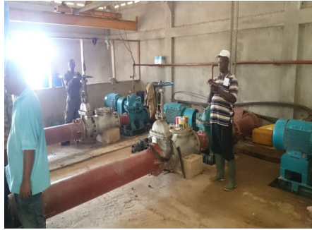
GIDA Irrigation Pumping House showing the Manager-in-Charge
