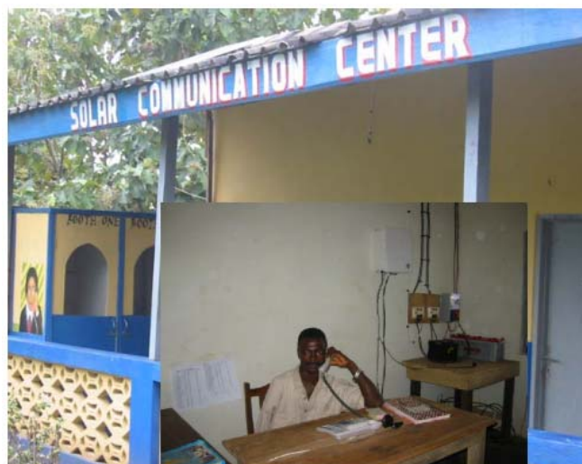
Fig 3.12: Solar System for Communication Source: Energy Commission, 2011
